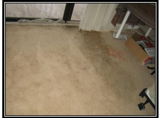
Stains on the carpet show an area that is always wet.
