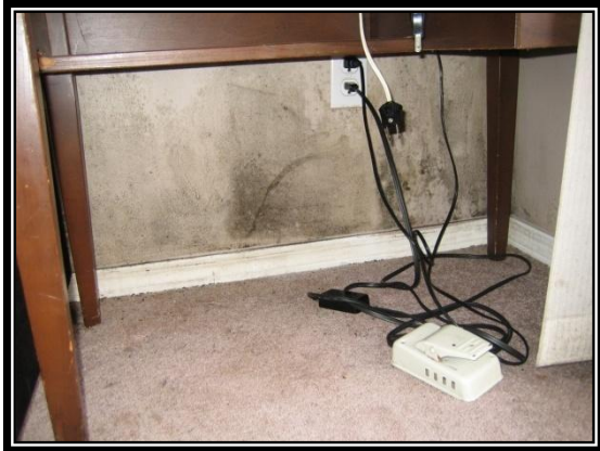
Black mould covers the wall in part of the living room.
